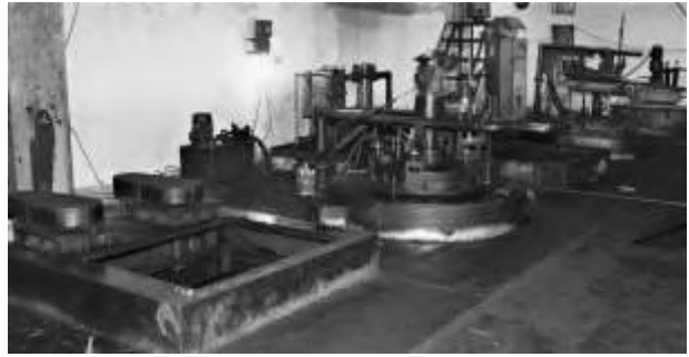
GAS CARBURIZING FURNACES
